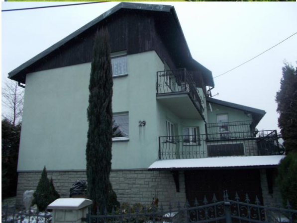
Fig. 1. The walls of the building as an extension of the foundation walls (Foto: M. Buško)
